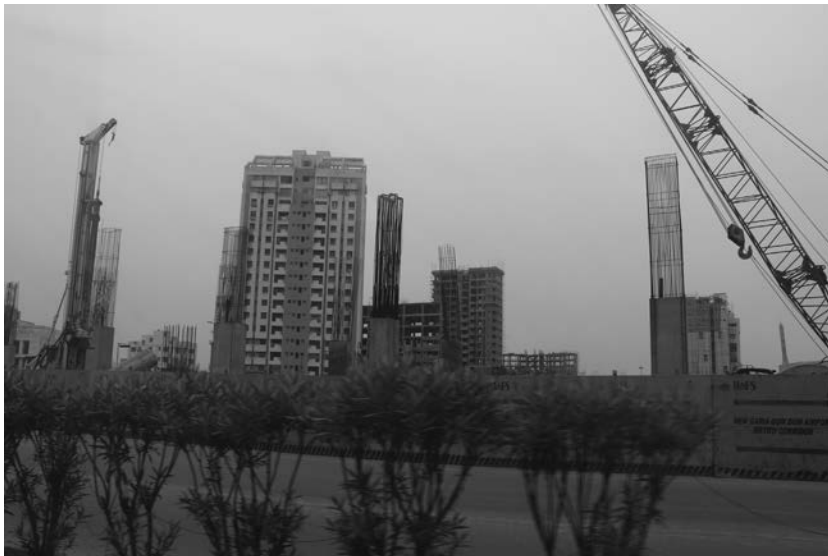
4.10 Rajarhat, district 5, New Town, Kolkata, India. Source: Photo by Orit Halpern, March 13, 2016.
